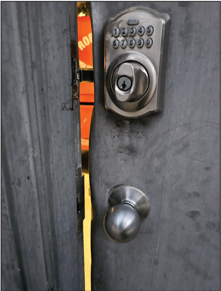
Forced entry marks remain on the fire station's metal door, which firefighters worked to repair despite running on little sleep. Photo by Fire Chief John Stull
