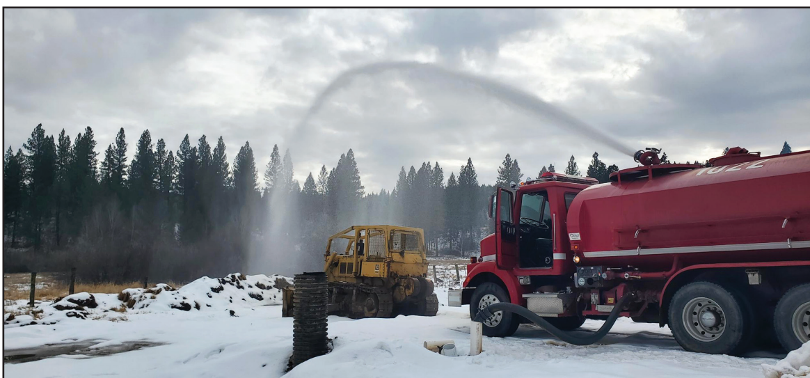
Water will be provided during the winter for fire suppression. Photos courtesy of Placerville Fire
