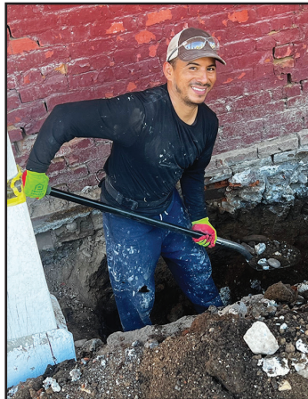
Trained brick layers dig up artifacts in the foundation of the Mercantile.
