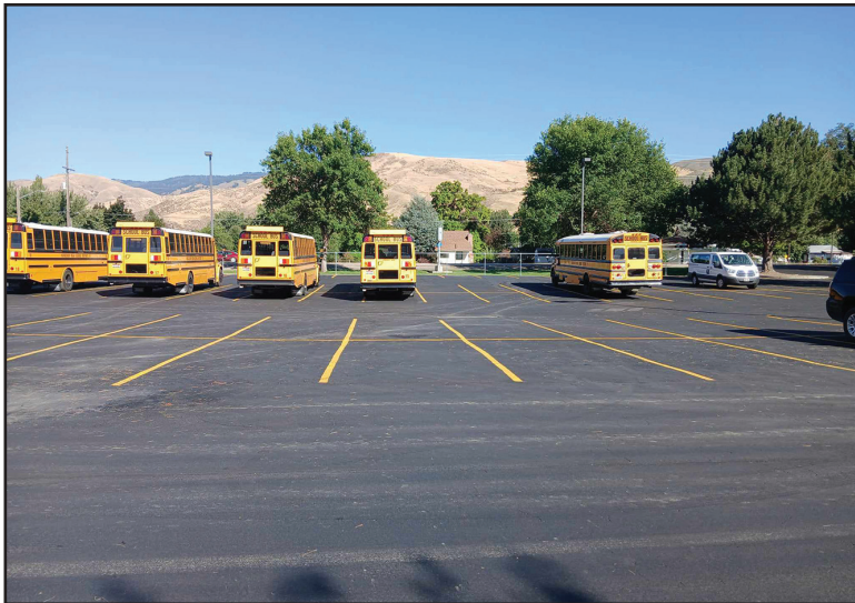
The Horseshoe Bend School District received an exterior facelift over the summer. New asphalt and, thanks to the state's SOF Grant, perimeter fencing that is currently being installed. Photo by Tracy Koslosky
