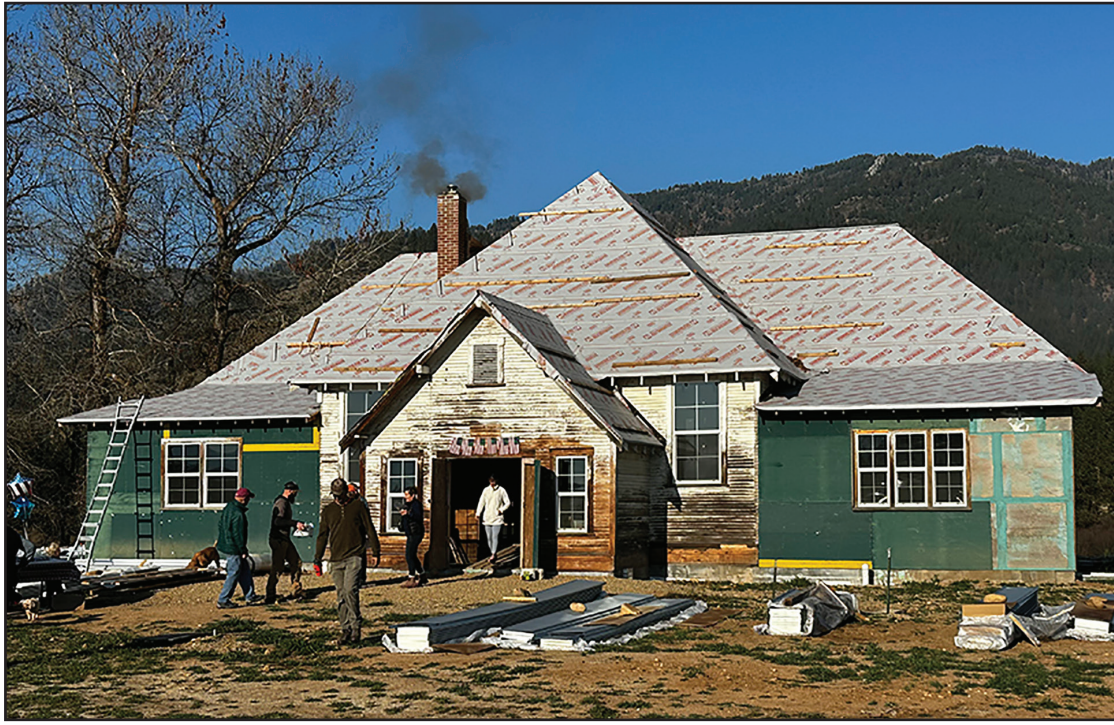
Slow and steady progress is being made on the old schoolhouse, converting it to become a home with indoor plumbing and electricity. Photos by Linda Ruppel, DDS
