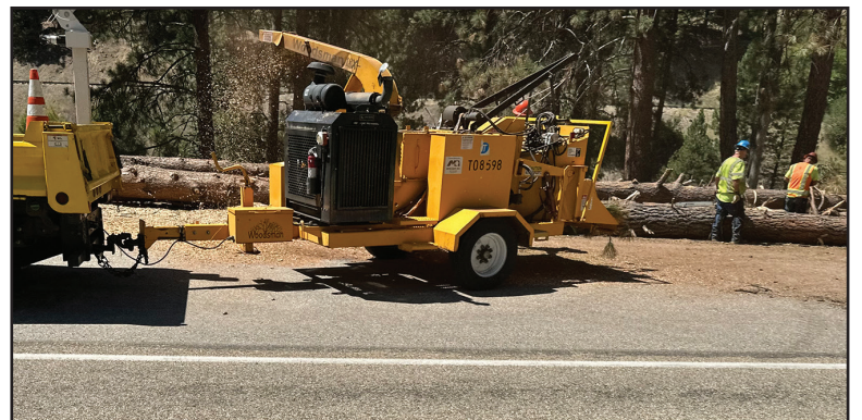
Last week the dead tree removal project got underway. Work will continue for several weeks on Hwy 55 between Banks and Horseshoe Bend, on Mondays through Thursdays. Photo by Linda Ruppel, DDS
