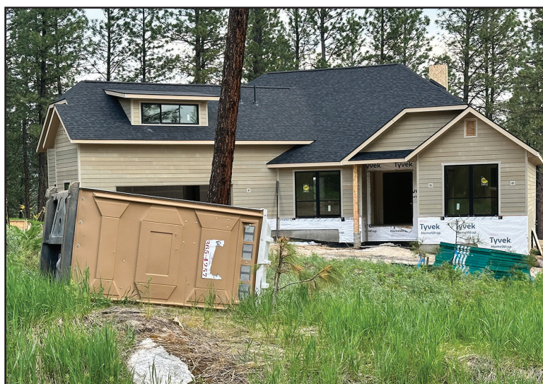
The winds were so strong that they even tipped over this porta-potty, which this photographer was not willing to investigate further.
