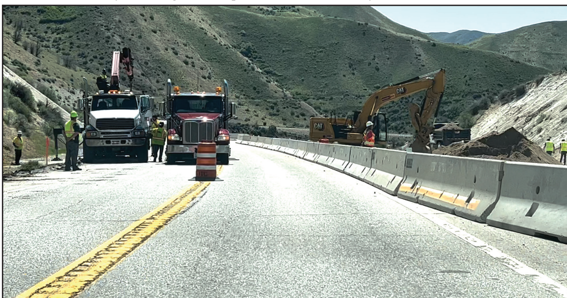
The new construction for the wildlife overpass on Highway 21 has begun and crews have one lane closed. The speed limit has been reduced to 25 mph.
