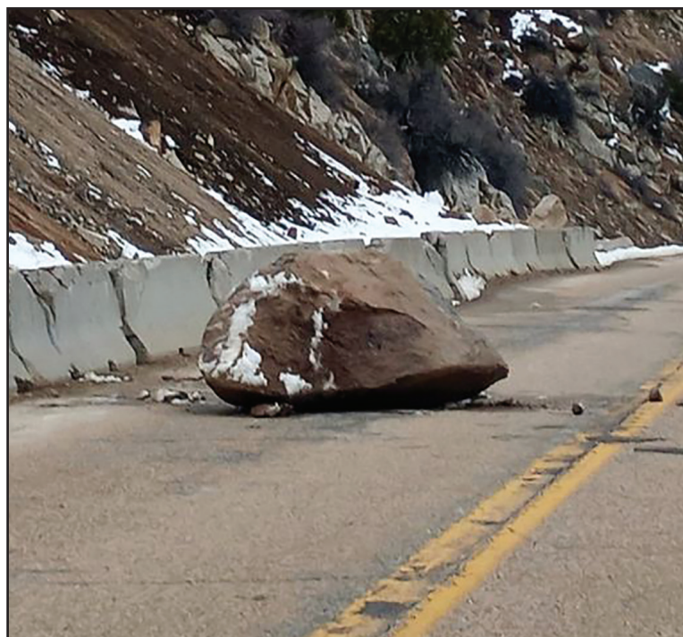
On Sunday, March 12th, this boulder rolled into the roadway. The boulder covered almost the entire lane and was located just prior to Pine Flats Campground on HWY 17 at about MM 28.
