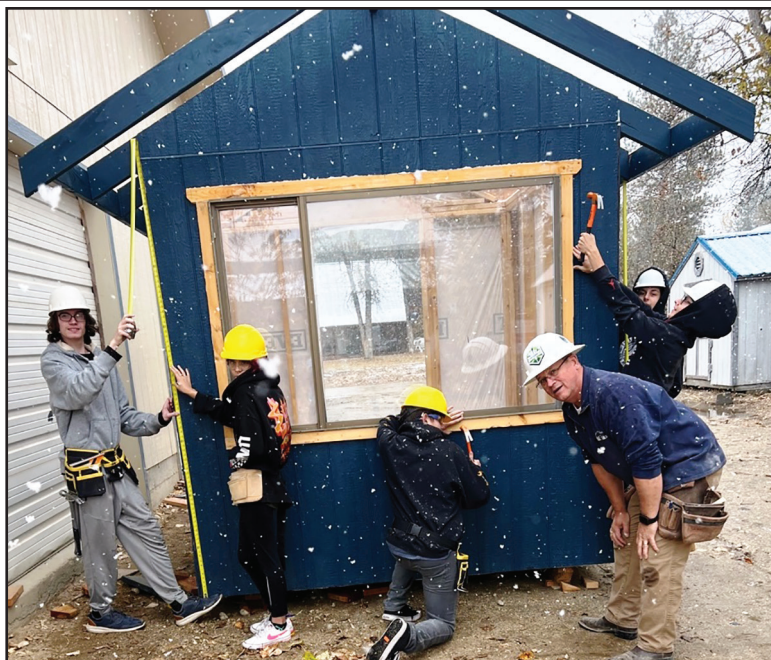
The High School Construction class was working on the ticket booth in the snow. From left to right, Shawn Lasalle, Sierra Genovese, Dylan Berger, Tom Standerwick, Charlie Culzer, and Wyatt Thomas.
