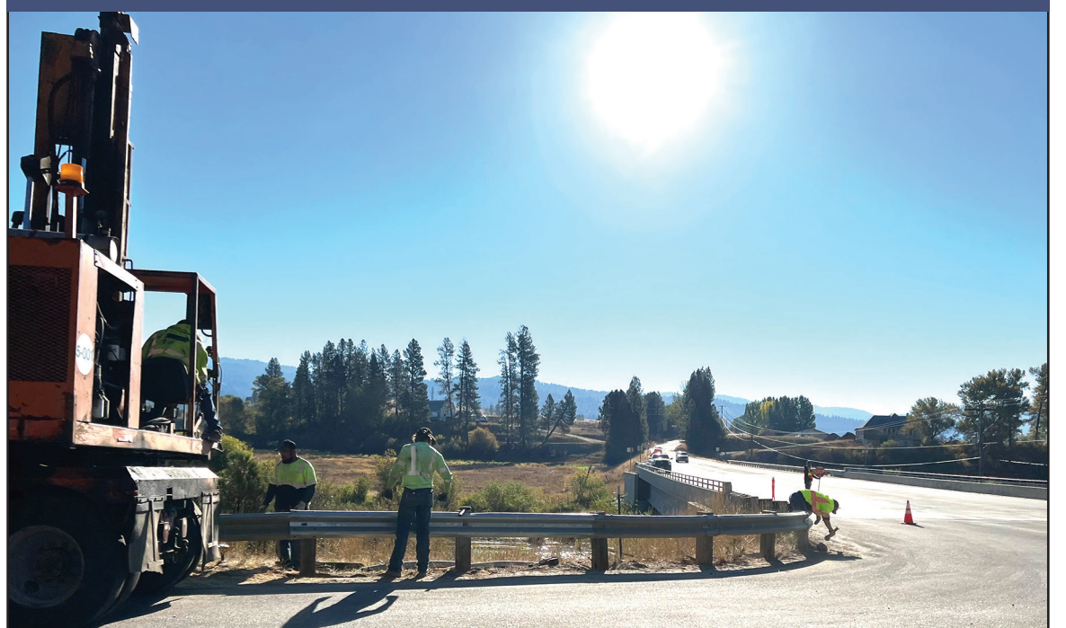
Nobody knows who bent the railing several weeks ago, but on October 3rd it was finally repaired. The accident was never reported, although the rail likely saved somebody from going into the river at the corner of Hwy. 17 and Middlefork Rd.
