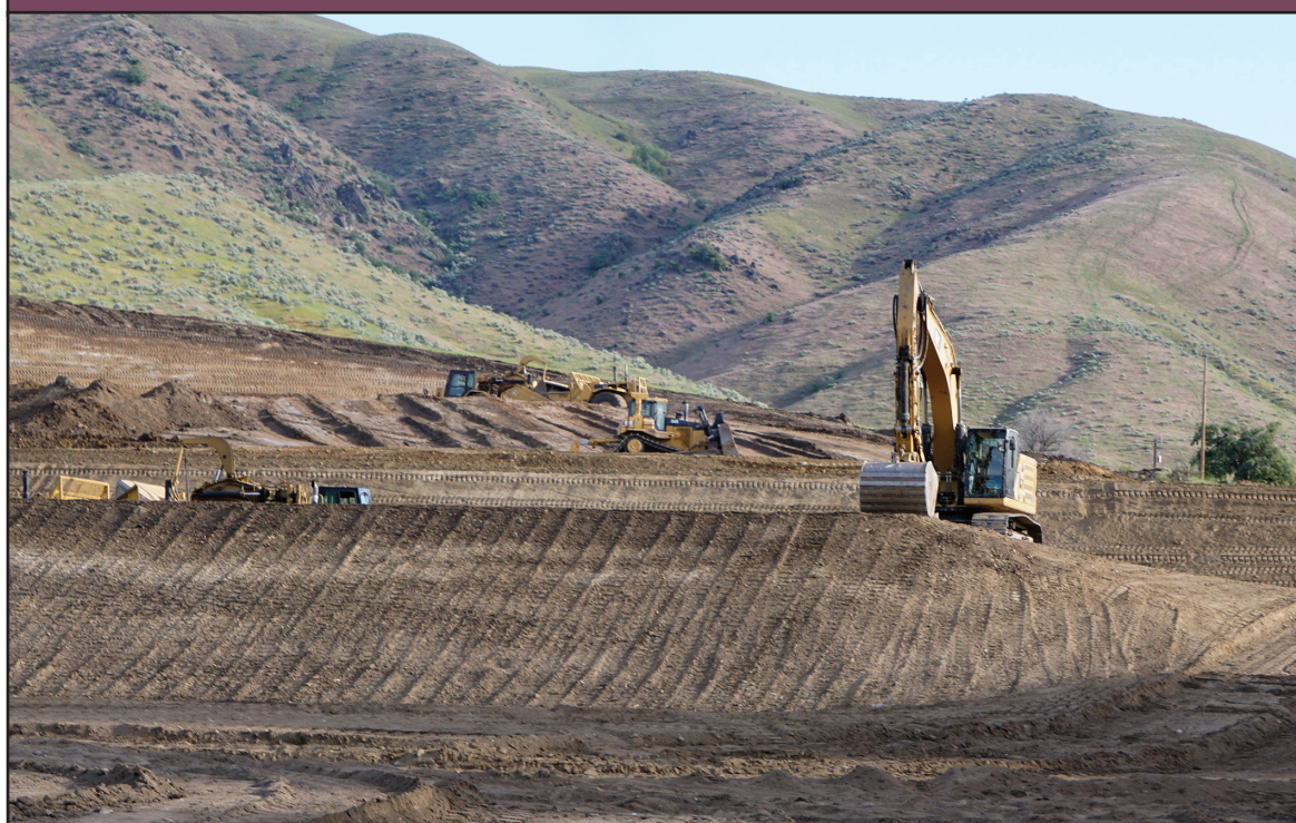
They're breaking ground and moving earth at the new Deer Valley Subdivision in Horseshoe Bend. The project has left the hands of David Bailey & Trilogy Development and is now a Corey Barton Homes project. Located on Highway 55 just north of Highway 52, the development will put approximately 140 single family residences and townhomes on 20 acres of land. Photo by Tracy Koslosky
