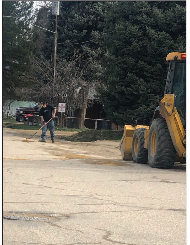
April showers brought lots of "potholes" to Idaho City streets. The Idaho City Public works department has been busy filling them with sand every time it rained. Gene Bettys works on Main Street shoveling sand into holes to stabilize roads.
