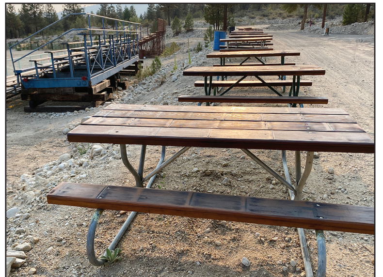
The bleachers were fixed with a sturdy foundation. The tables were redone with redwood from the water tower, then oiled beautifully. The upper area was leveled for spectators and vendors.
