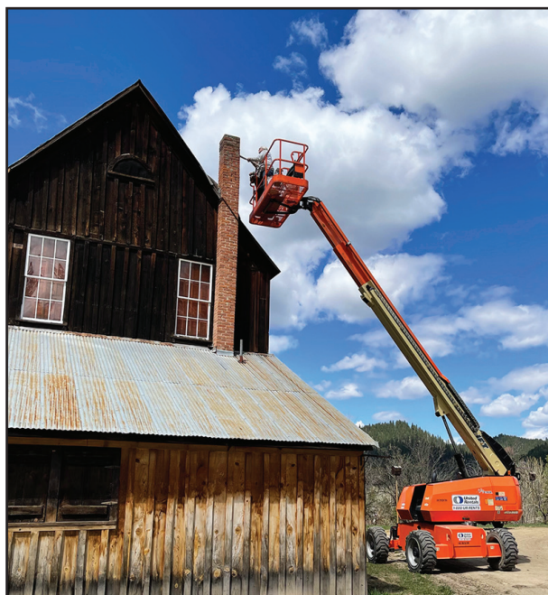
A crew repaired the Odd Fellows Building last week. This picture, taken by Barbara McClaim, shows how the Historical Foundation used a bucket to repair the chimney. Inside the bucket and doing the work were Charlotte Watson and Roger Jackson. Photo by Georgene Thomas
