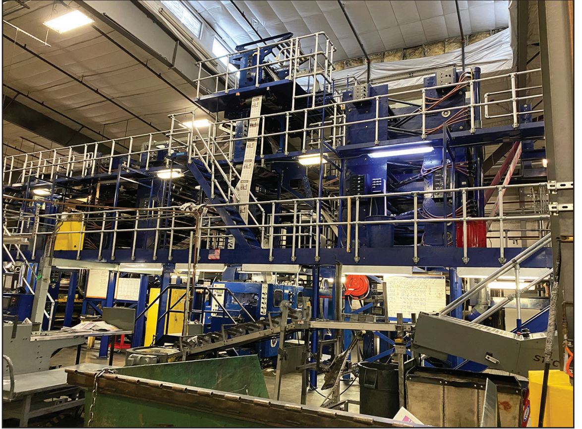
Raising the ceiling and moving the printer to its new location within the same facility, the press now extends another half story up, bringing it to a height of two and a half stories.
