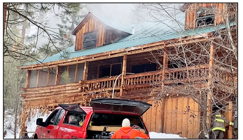
The house received extensive smoke damage, but appears to be repairable.
