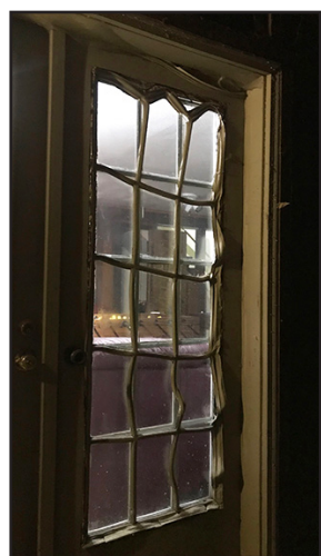
The fire melted the plastic within the French door on the house.
