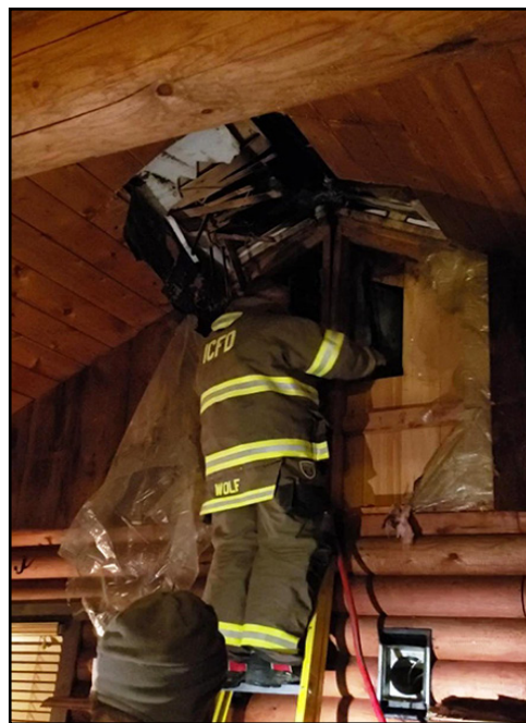
Idaho City Fire was quick to respond and put out the fire with minimal damage to the home.
