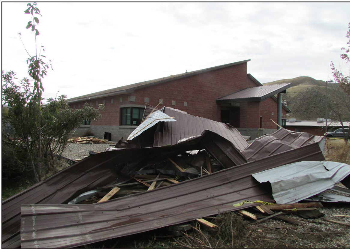
Horseshoe Bend's middle school metal roof ripped off during a windstorm. Photo by T. Koslosky
