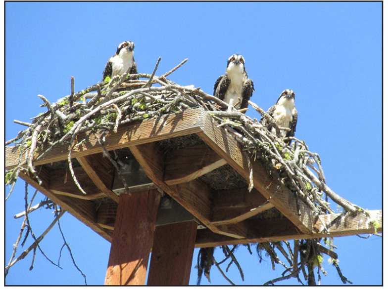
Osprey platform set up by Idaho Power to keep nesting material from arcing across the power lines. These fledglings have since spread their wings and left the nest. Photo by Eileen Capson
