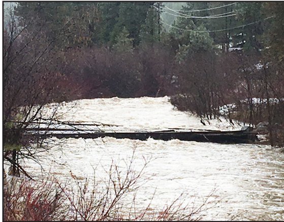
Bridge located south of Idaho City is nearly submerged.
