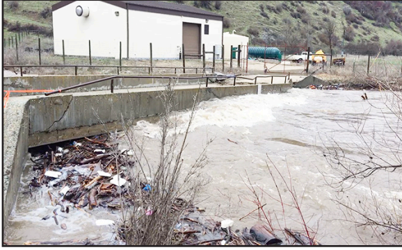
Robie Creek Road bridge was damaged, due to a high volume of spring runoff.
