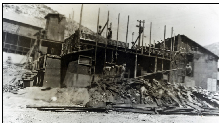
The store after it burned in a fire. It was rebuilt at the same location. Photos courtesy of the Idaho State Historical Society (ISHS)
