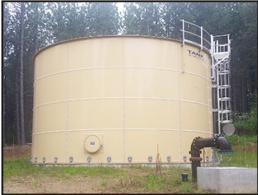
City of Crouch Water Tank - submitted by Mountain Waterworks
