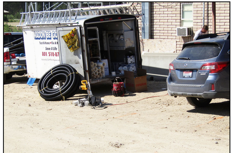
Radon gas professionals from "Radon Be Gone" arrived Monday morning to work underneath the Sheriff's Office installing a ventilation system. According to Health & Welfare, "Radon is a naturally occurring radioactive gas that comes from the breakdown of uranium in the soil. It is a colorless, odorless, tasteless and invisible gas." It is also said to cause lung cancer.
