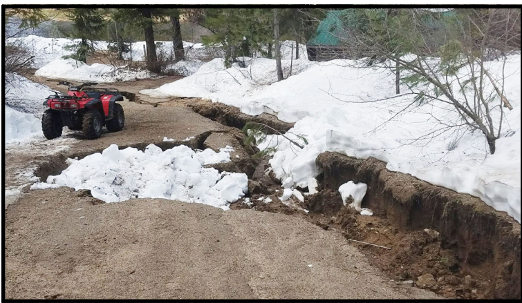
A small subdivision nine miles north of Crouch has a road that washed out due to snow run-off. The crevice is around 300ft long and there is a sink hole in the road also. One full time resident had to evacuate since the road is not passable except by a ATV. Runoff will continue for quite some time and homeowners are trying to figure out what work will need to be done. Photo by Janet Juroch
