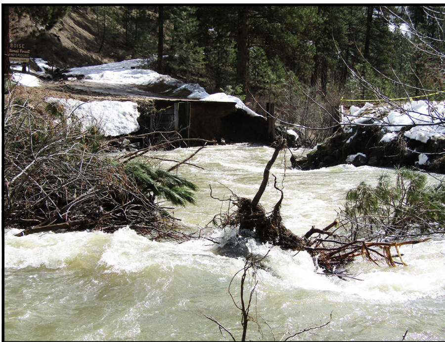
March 25th The bridge was too badly damaged for it to be repaired. Gardner Construction was hired to take out the decking.
