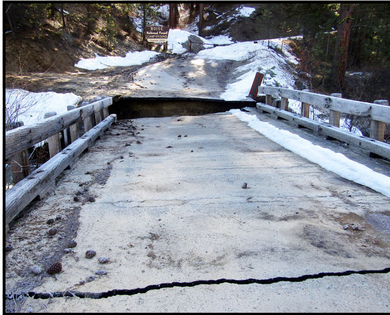
March 23rd Photo of Greyback Gulch Bridge. A tree had caused the water to be diverted and undermined the bridge. Photos by Eileen Capson
