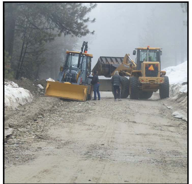
Bear Run Road was washed out with the heavy rains on Thursday morning. Boise County and Idaho City employees blocked the road leading to Duquette Subdivision to repair the deep ravine carved out by a stream of water.
