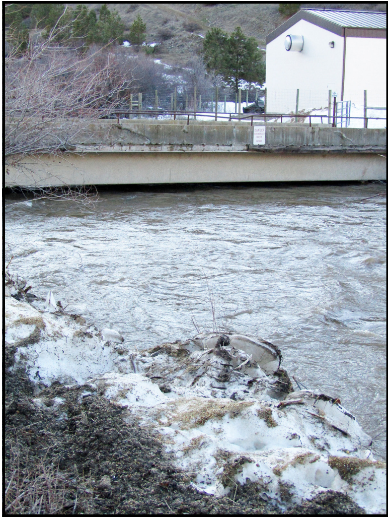
High waters come close to flooding and further erode around bridges. This bridge is located on Robie Creek Road and serves as a load bearing bridge for large trucks.
