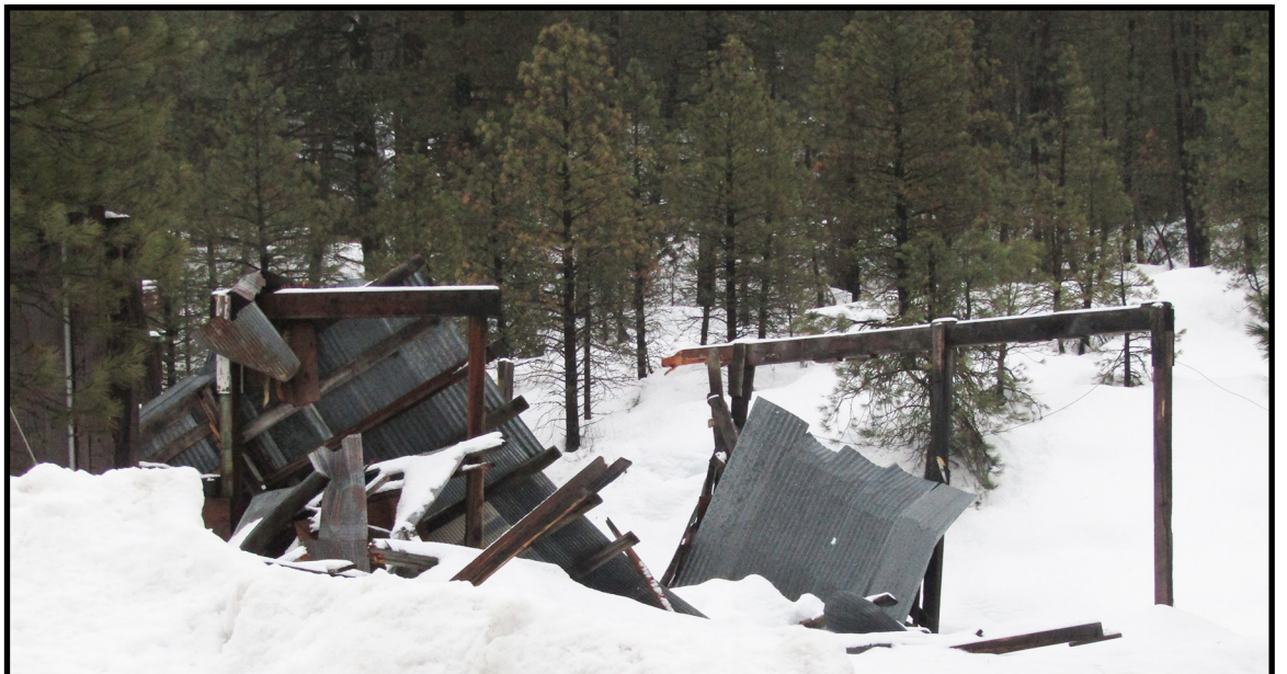
An increase in snowfall, doubled with cold temperatures, maintained a heavy weight upon rooftops, over the past several months. This one finally succumbed to the weight and collapsed. Luckily, a warming trend is now melting the snow. Photo by Eileen Capson
