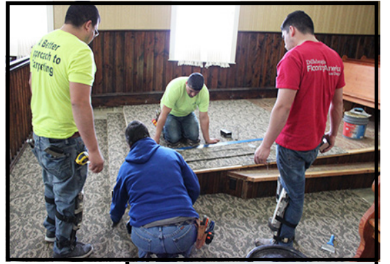
The crew with BCI have been working diligently, on the weekend, to have the courthouse remodel completed by the end of the month. Photo by Eileen Capson
